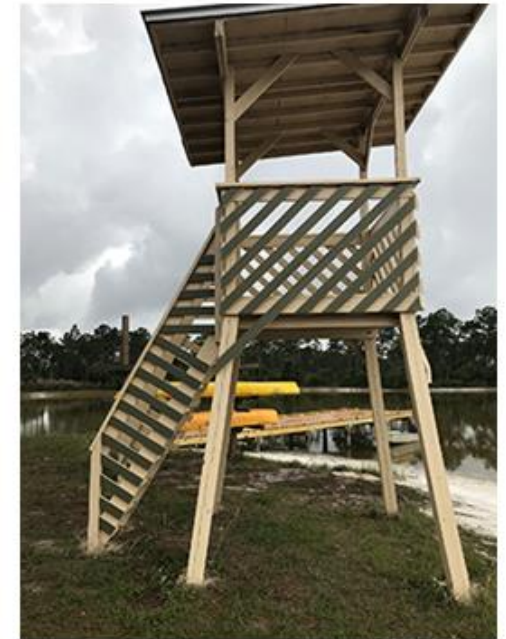
Photos of the completed Bridge, Kayak Racks, Boat Dock and Lifeguard Tower on the Camp Miles Adventure Island
